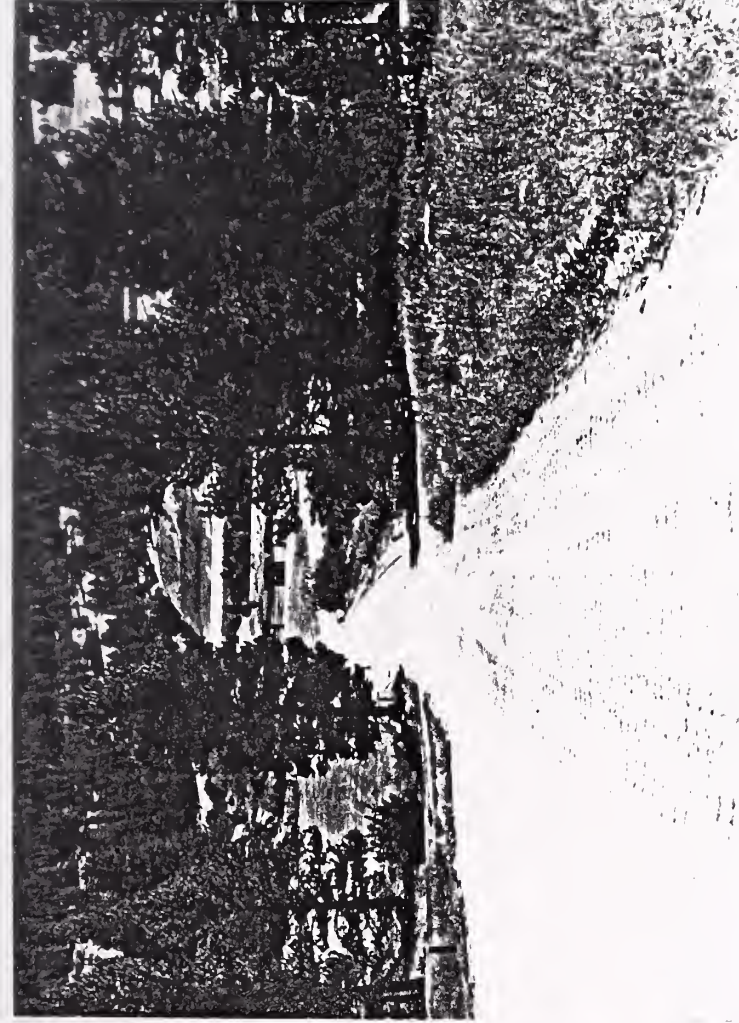
FOREST PARK DRIVE EAST BOUND MID SECTION (NOTE WASHBOARD)
